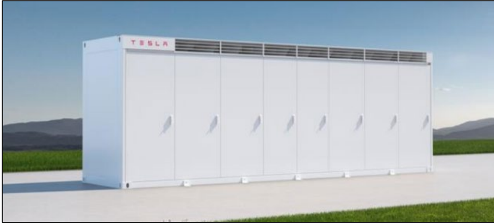
Figure 11: Image showing a typical BESS.
